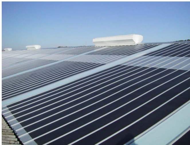
Figure 5 Typical Laminate Solar Installation on Metal Roofing (Uni-Solar)
