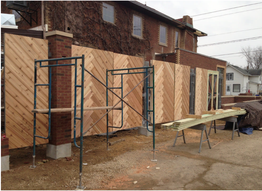
Proposed Fence Style for Seating Area; Current fencing on west side of building
