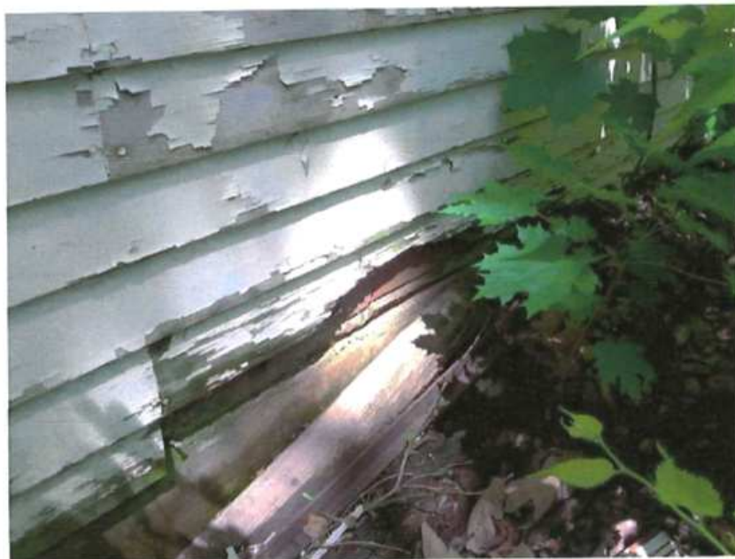
rot: wood siding (localized area)
