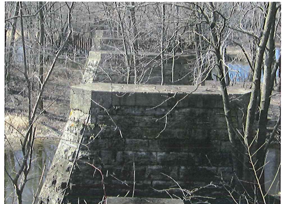
Existing bridge abutments over Bass Creek on the southeast side of Afton.
