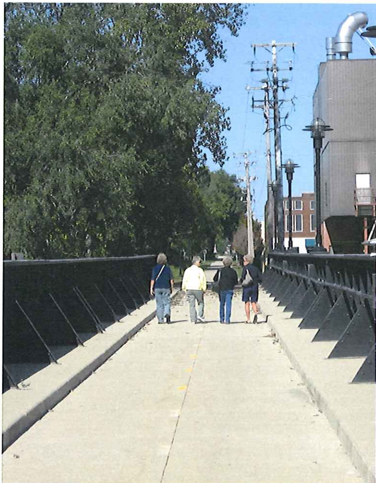
Footbridge over the Rock River in the City of Beloit. This is a segment of the 5th Street Trail running from the Wisconsin-Illinois State Line to Krueger Park.
