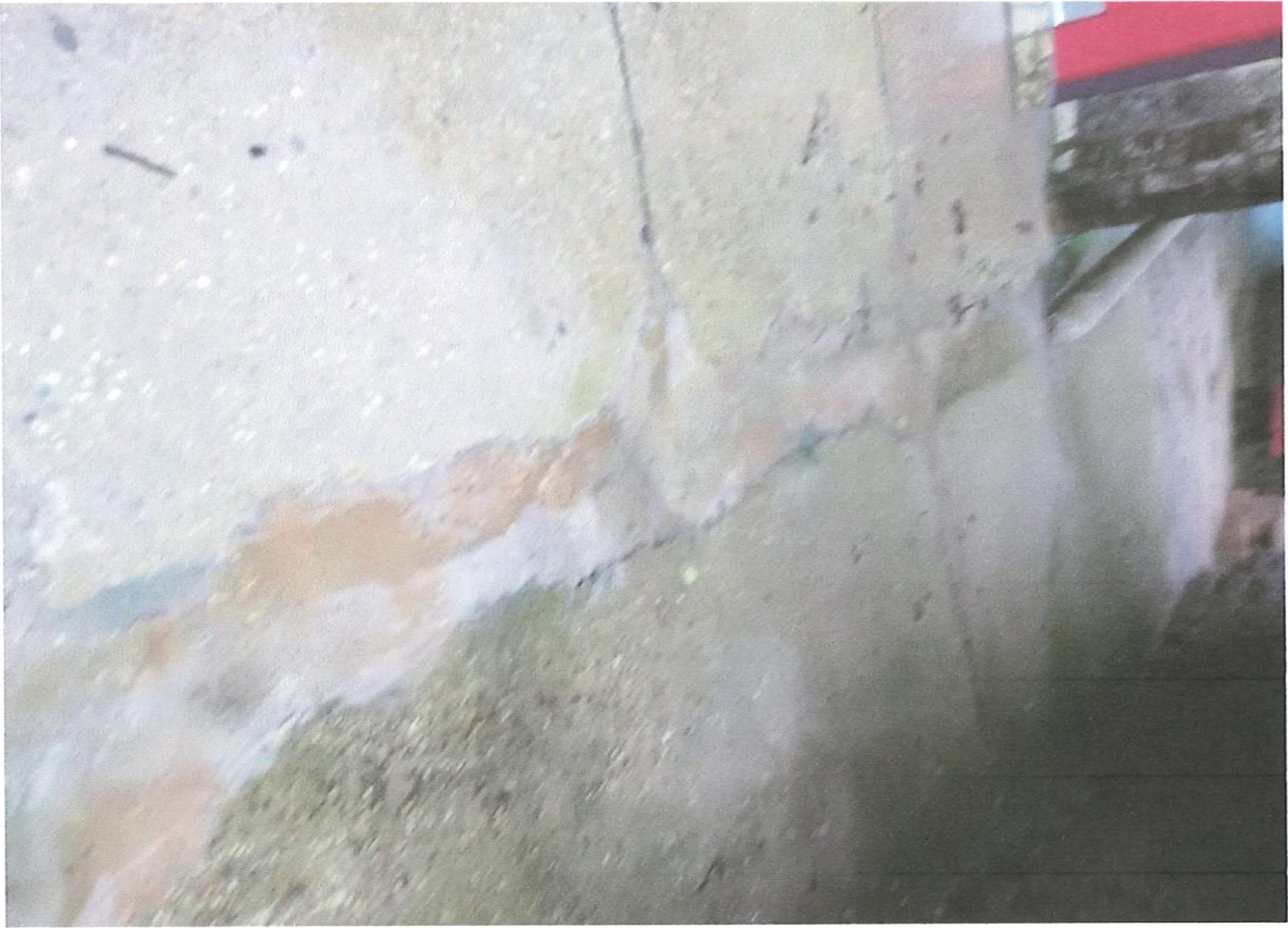
WEST SIDEWALK SHOWING CRACKING AND PITTING
