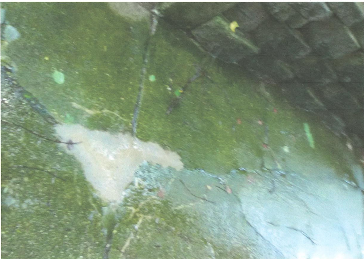
WEST SIDEWALK SHOWING WHERE AREAS OF MISSING CONCRETE HAS BEEN PATCHED
