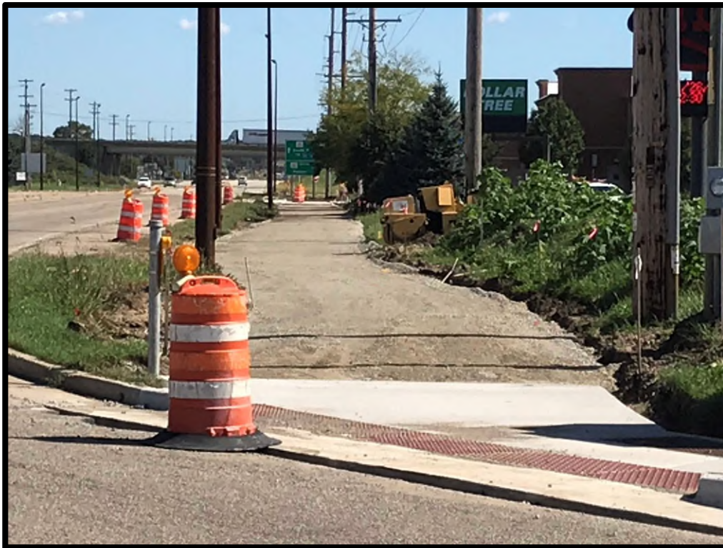
Rockton Road Bike Path shown under construction September 2019. ITEP award received in 2014. Illinois 251 Bridge in background currently planned for replacement in 2024.
