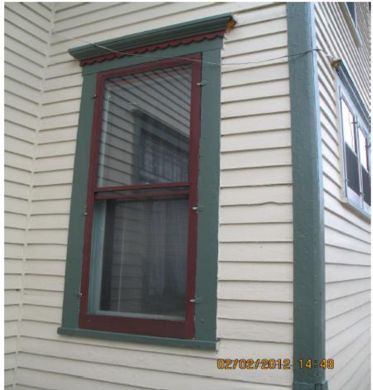
Lower window on northeast side of house that will be replaced.
