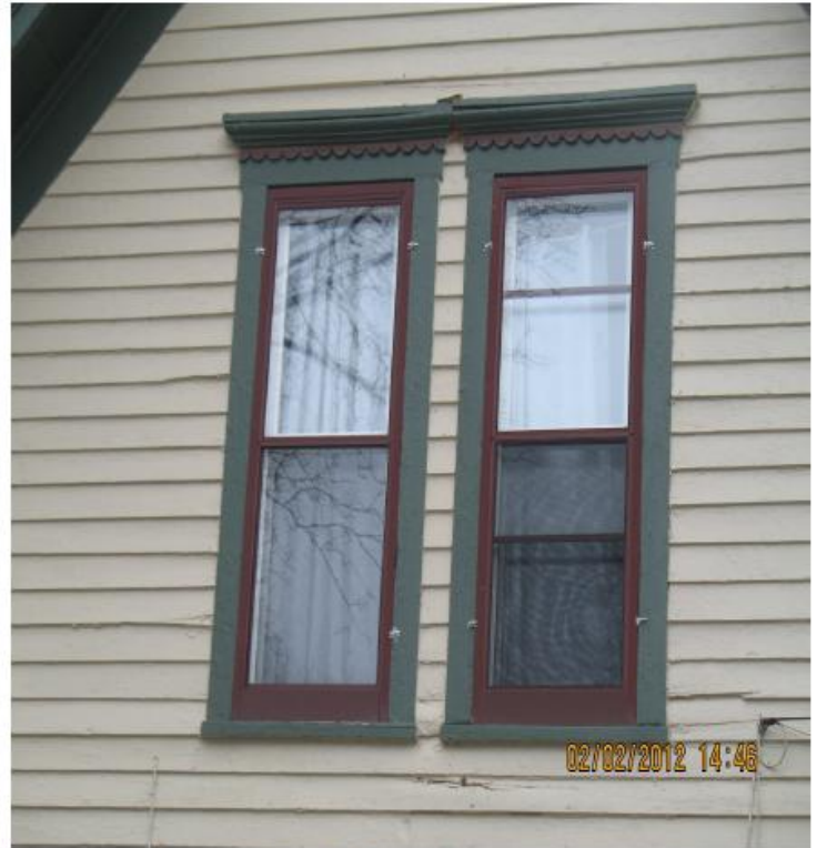
Upper windows on the south side of house that were replaced without a COA or Building Permit.
