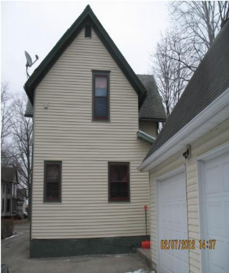
West side of the house ( rear of house). The lower window on left-hand side is location of window replacement.
