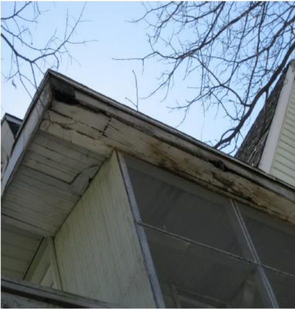
Rotten soffit and fascia boards on the northeast side of the property. Photograph taken by Code Inspector on March 30, 2011.
