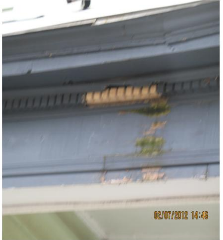
Replaced ornamental trim on veranda on the northeast side of the property.
