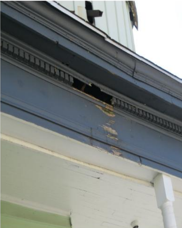
Missing ornamental trim on veranda on the northeast side of the property. Photograph taken by Code Inspector on March 30, 2011.
