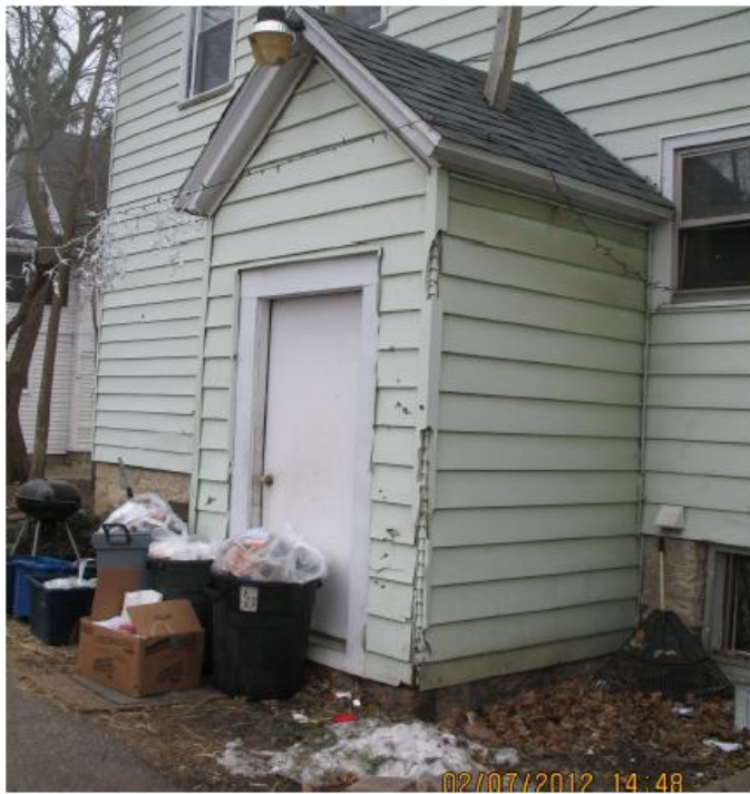
Damaged siding and trim on east side of the property.
