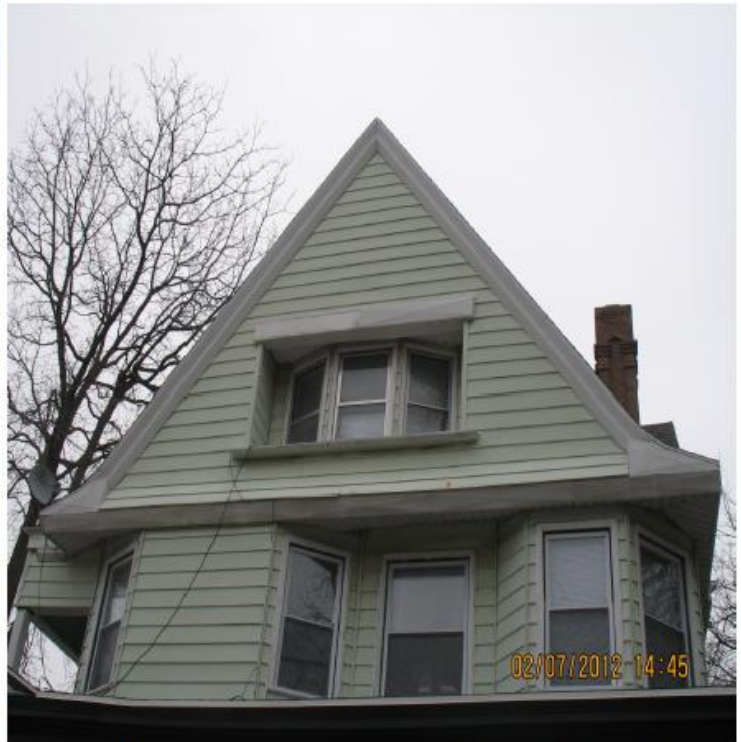
Removed bargeboard panels on gable located on the west side of the property.
