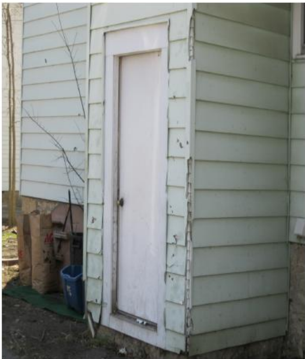
Damaged siding and trim on east side of the property. Photograph taken by Code Inspector on March 30, 2011.
