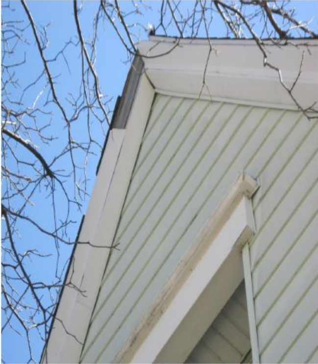
Missing bargeboard panel on west side of the property. Photograph taken by Code Inspector on March 30, 2011.
