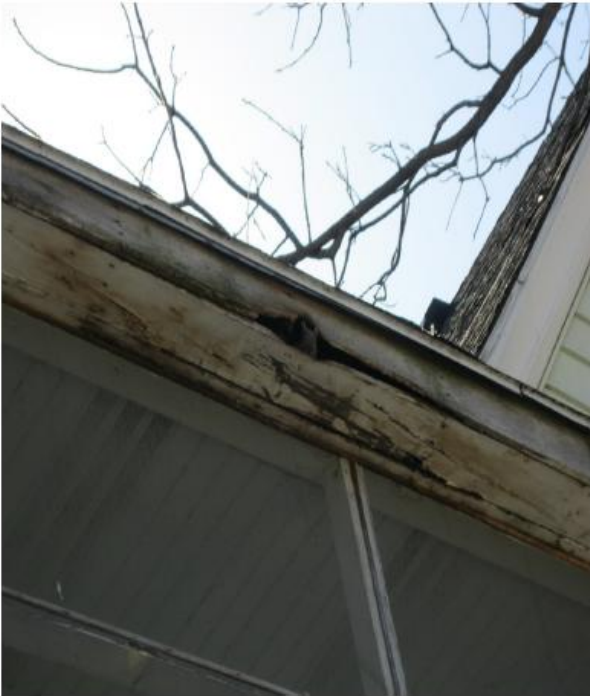
Rotten soffit and fascia boards with squirrel in hole on the northeast side of the property. Photograph taken by Code Inspector on March 30, 2011.
