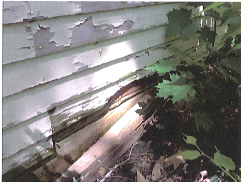
rot: wood siding (localized area)
