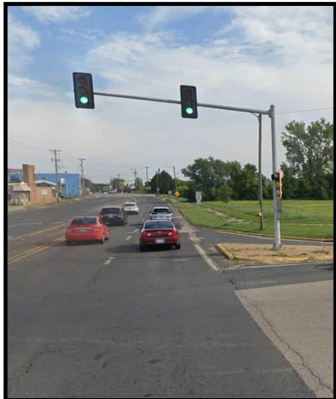
IL 75 at IL 2, looking north (note west-facing signal head missing covers)
